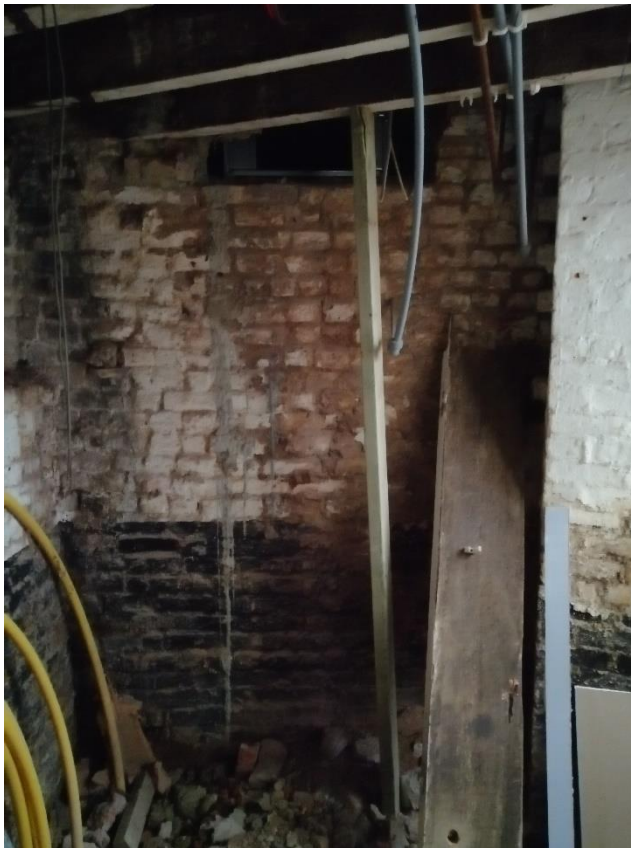
Figure 1 Photograph of untreated wall at lower ground level
